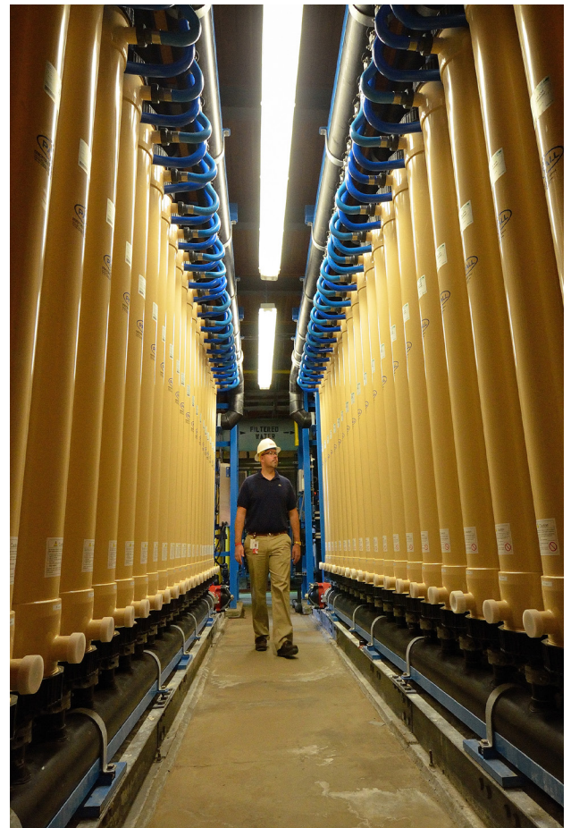
PWSA Microfiltration Plant located in Highland Park
