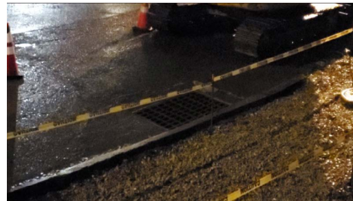
Twitter comment: “Credit where credit is due, especially given everything with COVID-19. @pgh2o fixed the catch basin here and so far there is no flooding. No snarky remarks. Just thanks to the folks who have been working hard out here. You are appreciated.”
