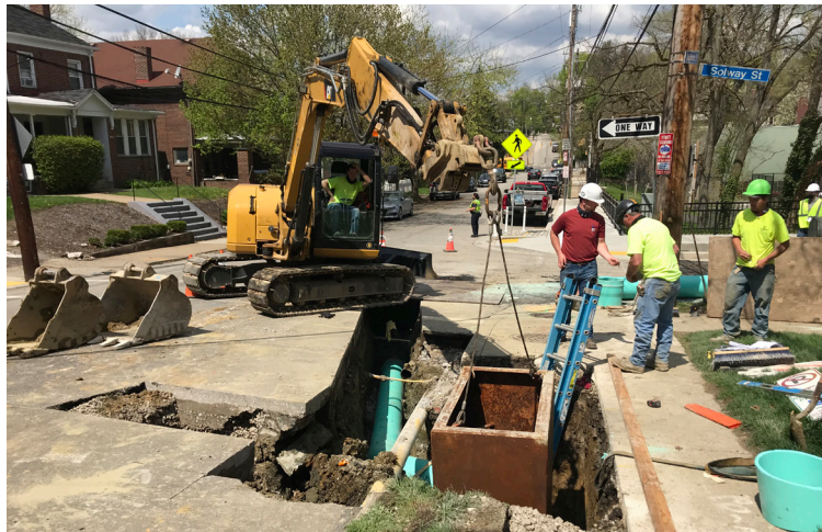
Construction crews have excavated the stormwater system at Wightman and Solway streets in Squirrel Hill. They prepare to install a catch basin into the system.
