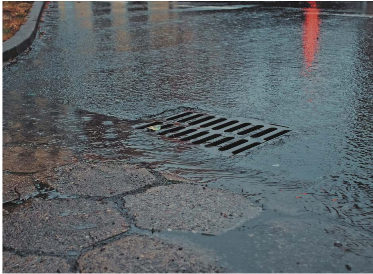
Community members are encouraged to report issues such as impaired storm drains, flooding, illegal dumping into sewers and basement backups. PWSA dispatch is ready to help 24/7.
