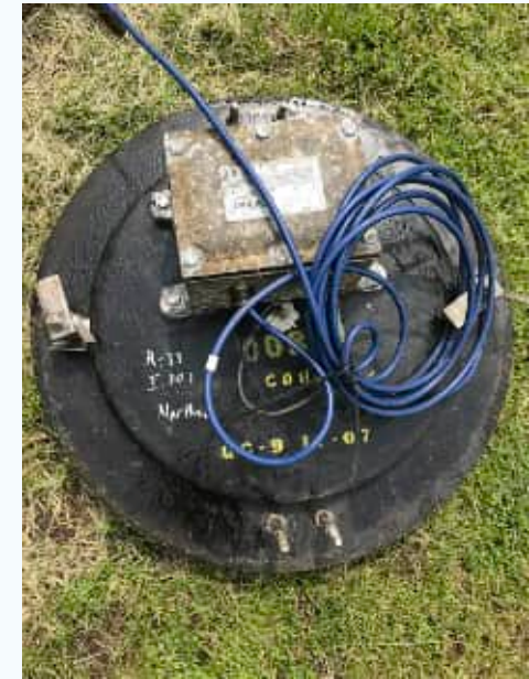
▲ The collection system in South Bend, Indiana, contains approximately 160 sensors, enabling real-time monitoring of flow and level measurements.
