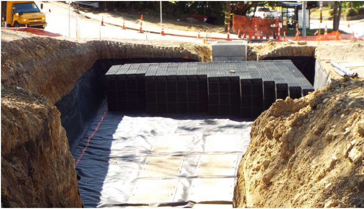
A retention tank at our Centre and Herron Green Infrastructure project detains stormwater and reduces the amount of water entering pipes.
